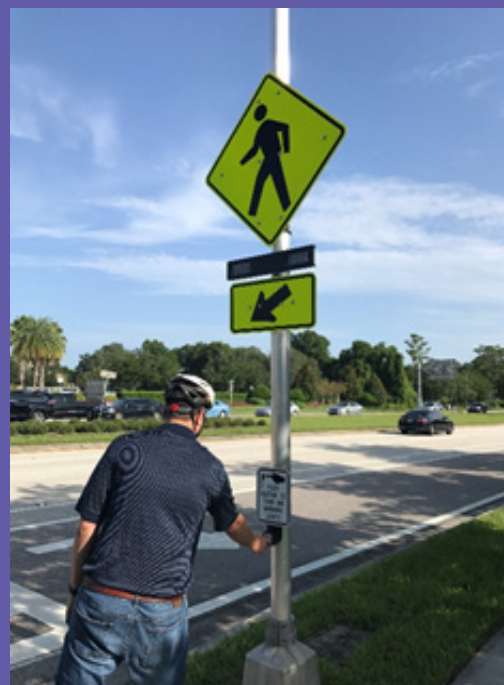
Bicyclist Activating RRFB- Controlled Midblock Crossing
